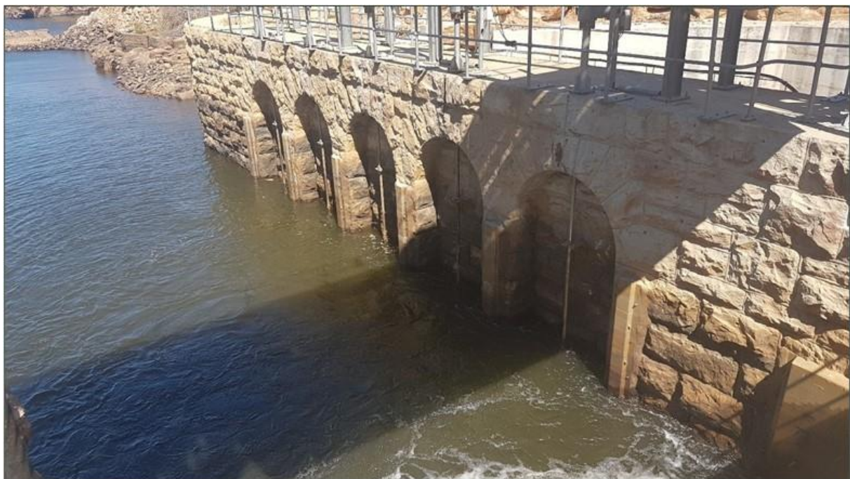
Figure 7-5: Bulshoek Weir outlet structure sluice gates
